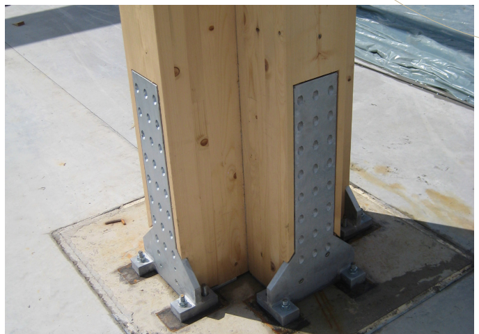
Cross support without steel plinth, in interior (no exposure to weather). Slanting screw connection and threaded connection of wooden parts. Anchor rod with thread in concrete or base plate with female thread integrated in foundation.
