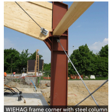
WIEHAG frame corner with steel column
